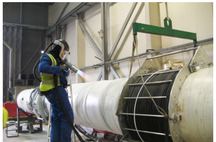
The above field joint is being flame spray coated with Plascoat® PP10.
